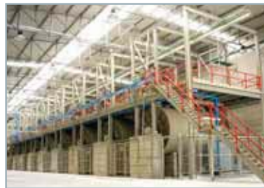
3 mulini discontinui - discontinuous mills
