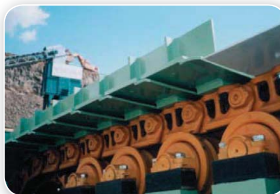
Apron conveyor chains, roller and buckets.
